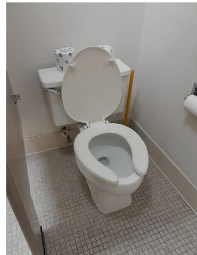
Figure 2 - Mezzanine Restroom Toilet
