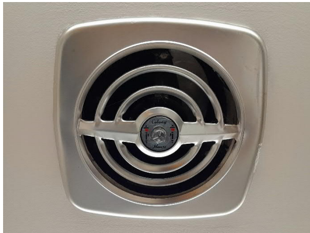
Figure 19 - Ceiling Mounted Exhaust Fan
