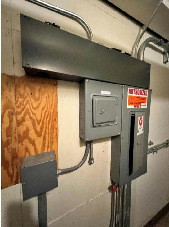
Figure 1 – Main Distribution Panel
