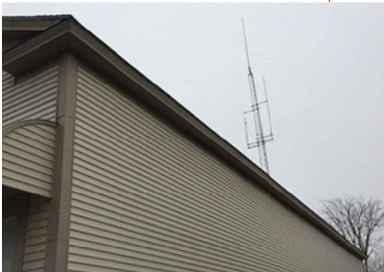
NO ROOF DRAIN, GUTTER, DOWNSPOUT
