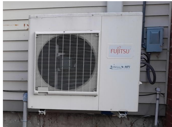
Figure 17 - Heat Pump Outdoor Unit
