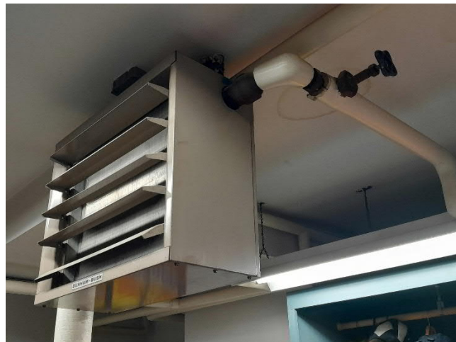
Figure 12 - Horizontal Unit Heater
