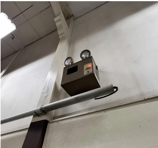
Figure 5 – Existing Emergency Lighting
