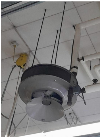
Figure 13 - Vertical Unit Heater
