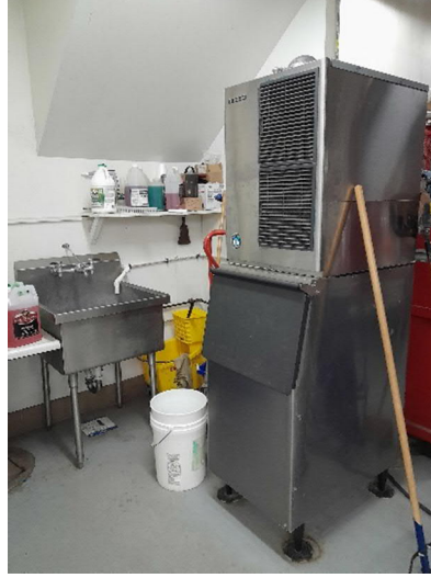
Figure 5 - Equipment Bay Service Sink & Ice Machine
