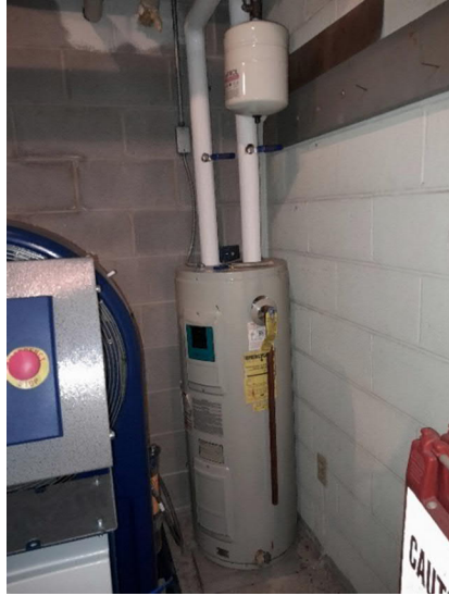
Figure 7 - Electric Water Heater & Expansion Tank
