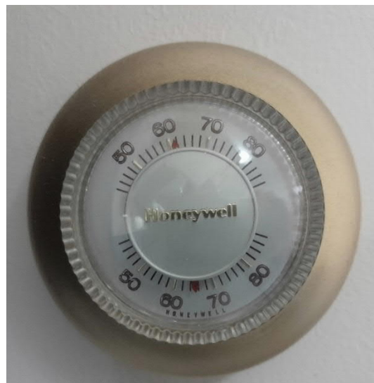
Figure 25 - Space Heating Zone Thermostat
