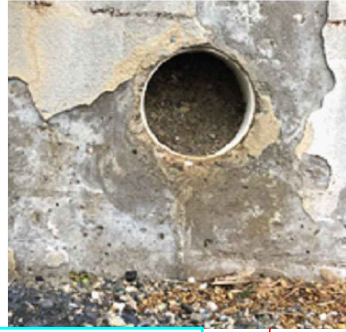
PLUGGED WEEP HOLES
