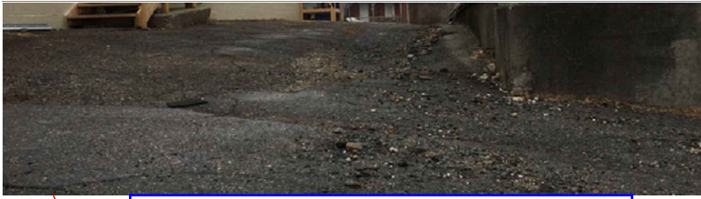
PAVEMENT UNEVEN AND DAMAGED
