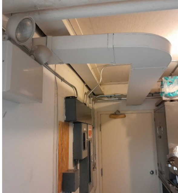
Figure 22 - Kitchen Exhaust Fan Ductwork
