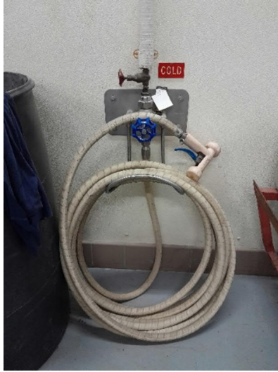
Figure 6 - Equipment Bay Hose Bib
