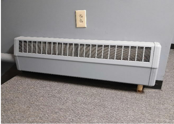
Figure 15 - Fin Tube Radiator Exterior
