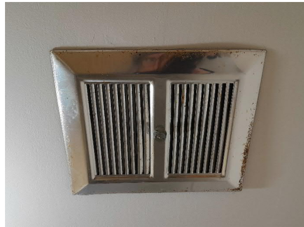
Figure 18 - Ceiling Mounted Exhaust Fan
