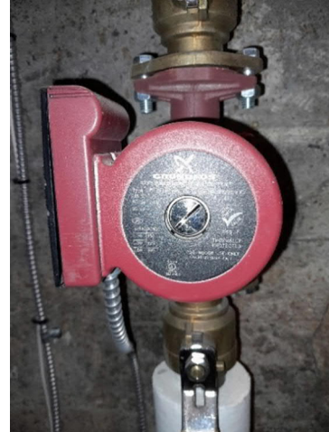
Figure 11 - Primary Circulation Pump
