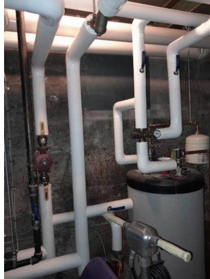
Figure 8 - Indirect Water Heater, Expansion Tank, Mixing Valve
