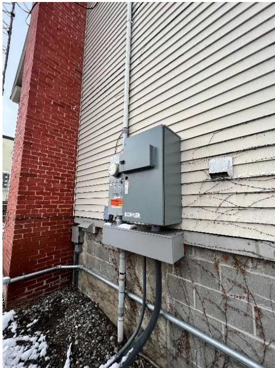
Figure 3 – Service Meter & ATS
