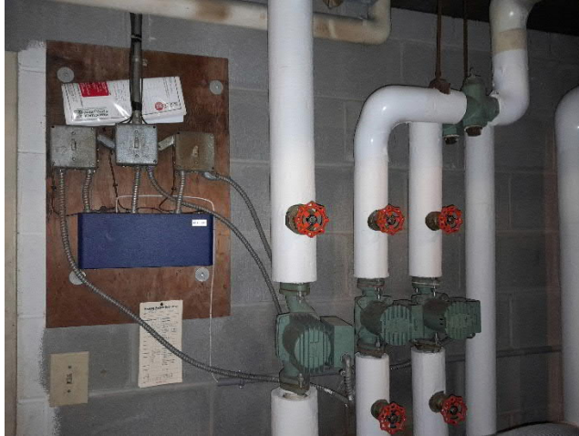
Figure 10 - Secondary Circulation Pumps
