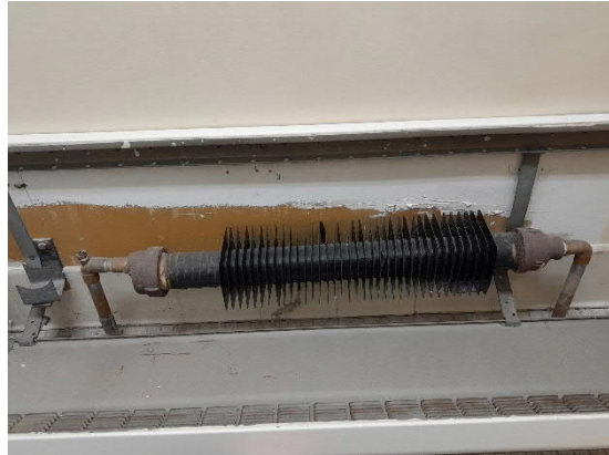
Figure 14 - Fin Tube Radiator Interior
